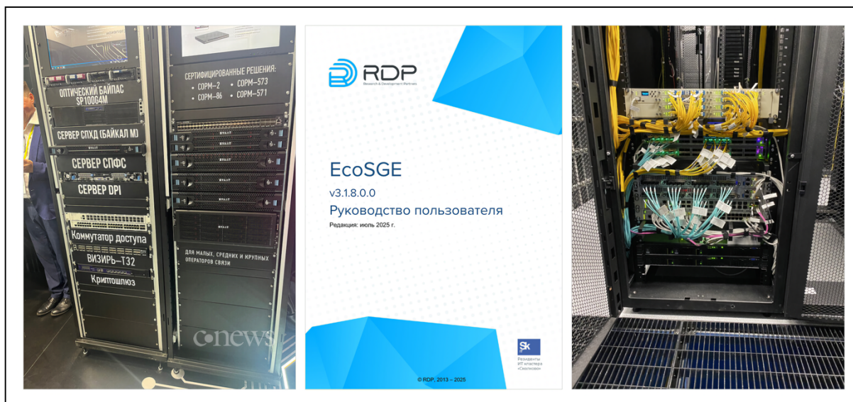
Figure 6: TSPU hardware: labelled server rack, EcoSGE DPI manual, and installation at ISP premises. Sources (left to right): CNews, 10 July 2024; RDP.RU; ISP practitioner documentation.
