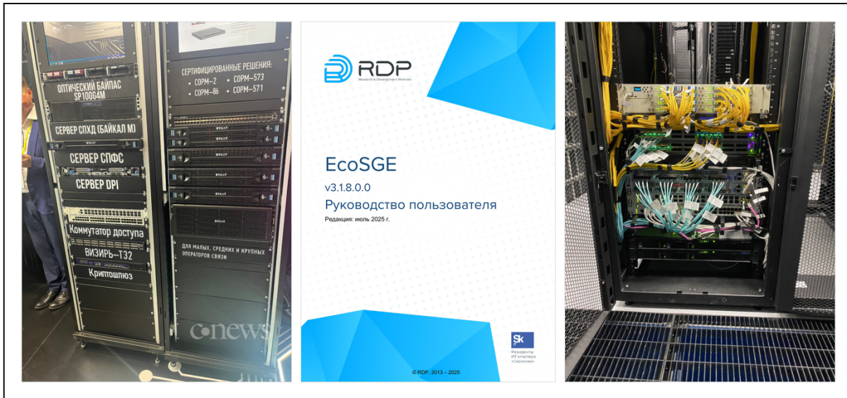
Figure 3: Deployed TSPU rack with labelled components (left), EcoSGE DPI platform interface (centre), completed installation at ISP premises (right). Source: CNews, 10 July 2024 (left); RDP.RU (centre); ISP practitioner documentation (right). 10, 11, 17
